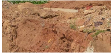
Plate 4. The collapsed culvert located at coca-cola road, Ilorin
